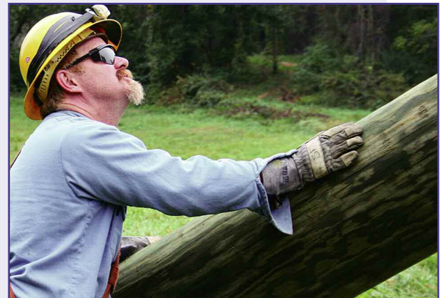
Lineman Brian Harber works to set a new pole and watches closely as the derrick truck begins to lift the pole into place.
