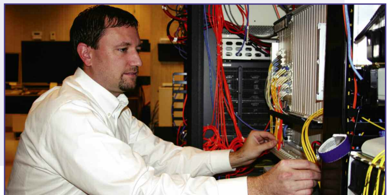
Network Supervisor Michael Parker makes sure that the fiber-optic cables are securely in place and working properly.
