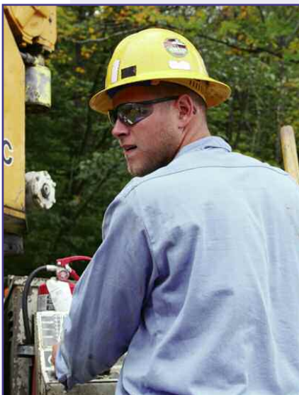
Lineman Josh Cunningham works the controls to the auger to dig a 10-foot hole for a new pole to be set.
